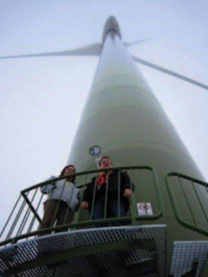
Andrew tours the 50MW Nuttby Mountain Wind Farm. It generates enough energy for 15,000 homes.
